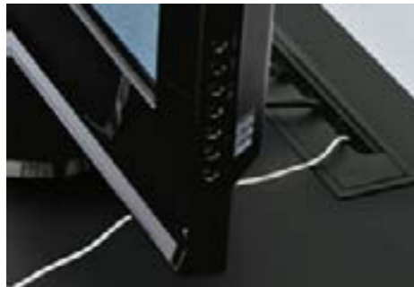
1 canalina passacavi / slotted cable gland
